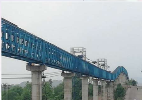
The Long Pipe Conveyor installed by Tata Steel at West Bokaro. (Credit: Tata Steel.)
